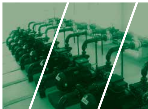
Boosting and Distribution of surface water
