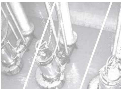
Wastewater Transport and Treatment
