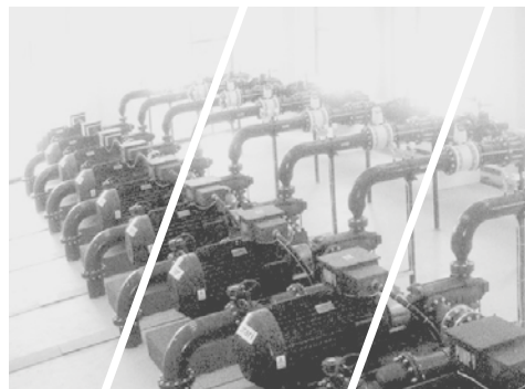
Boosting and Distribution of surface water
