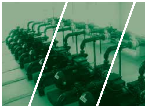
Boosting and Distribution of surface water
